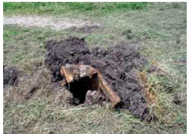
One of many items of debris encountered in the imported topsoil during remedial works
